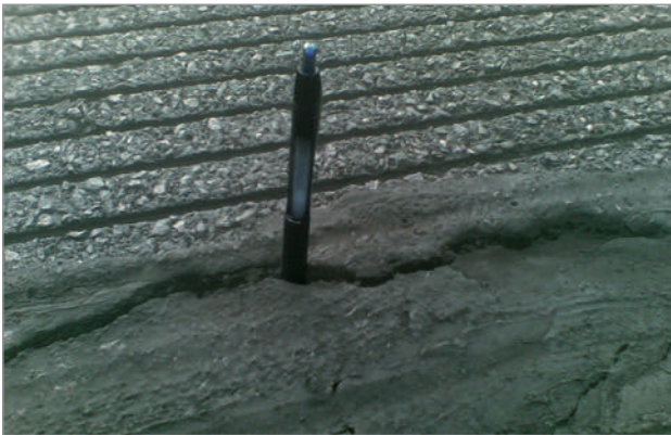
Wide crack (reflective crack) before rehabilitation works
